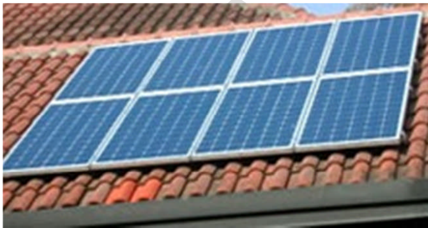
Photo 1. Example of Domestic roof PV System
