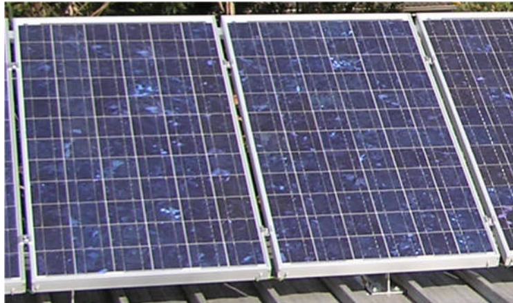
Photo A5. Multi-crystalline PV modules.
