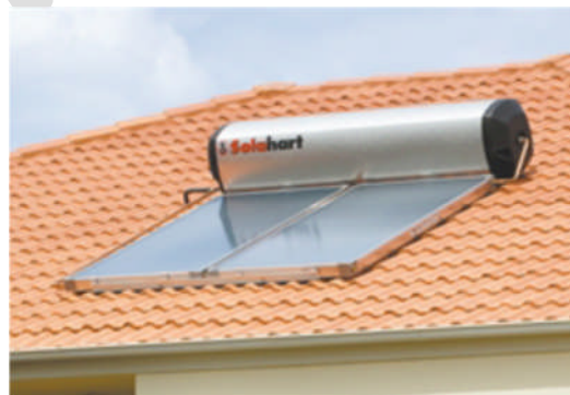
Photo A2. Solar thermal panels with storage tank.
