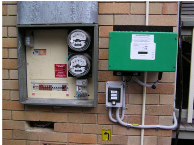
Photo A9. Example of Inverter installation adjacent to switchboard.
