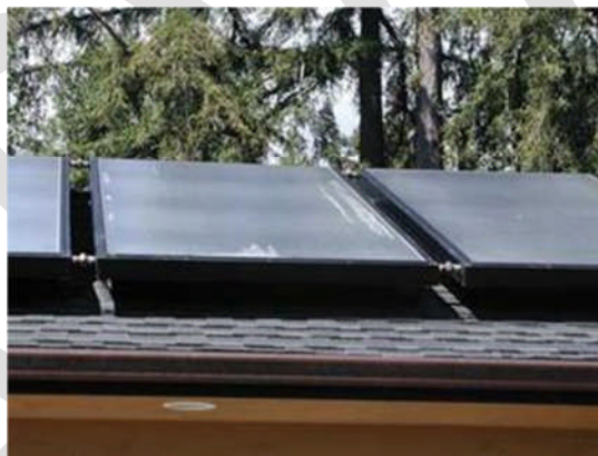
Photo A1. Solar thermal panels used for hot water
