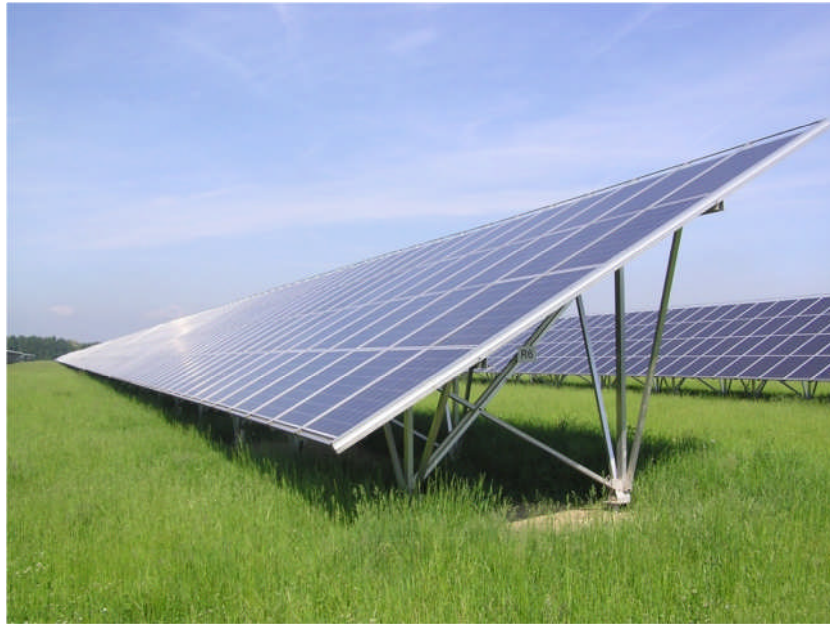
Photo 3. Example of Commercial Ground Mounted PV System
