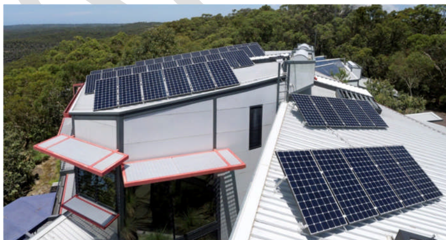
Photo 2. Example of Commercial Roof Mounted PV System (Photo courtesy of Sydney Solar Pty Ltd)
