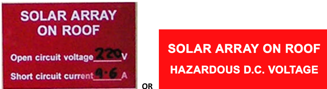
Photo 4. Example of Signage in Switchboard
