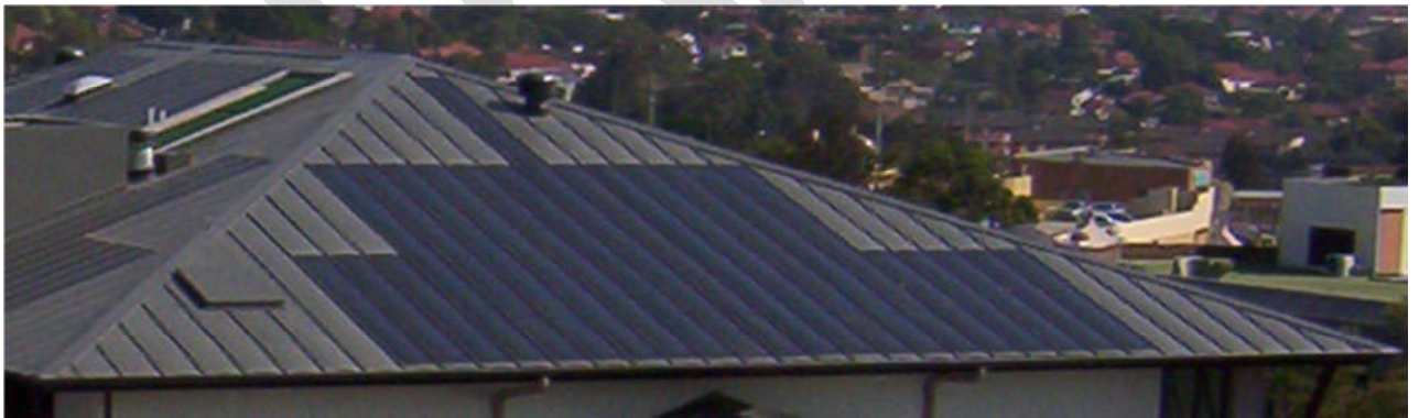
Photo A8. Amorphous modules bonded to metal roofing.
