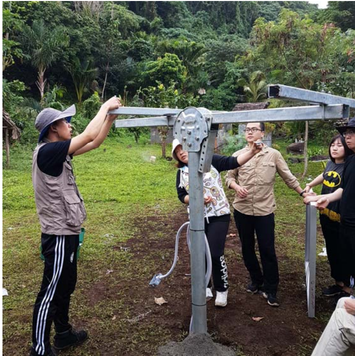
Fig. 1. The roof of the aid post at Uruwaren is shaded in the mornings so a pole mount was installed 25m away.
