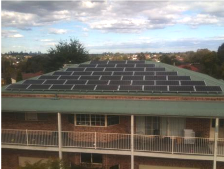
Silex Solar panels installed in Epping, NSW by Soltek Energy
