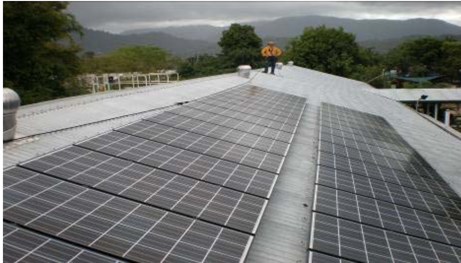
Figure 6: PV System at Edge Hill State School, Cairns. Photo: Ergon Energy
