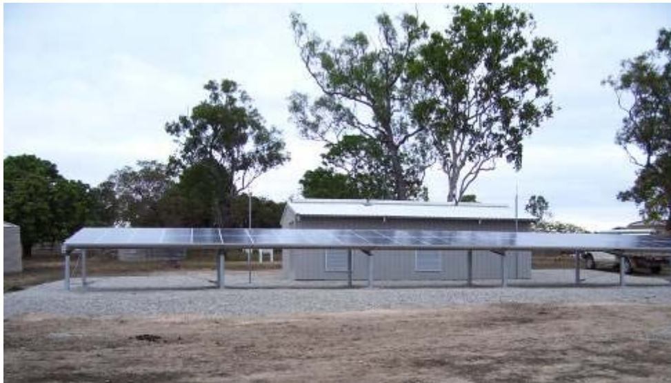
Figure 5: Bushlight system at Glen Garland. Photo: Ergon Energy
