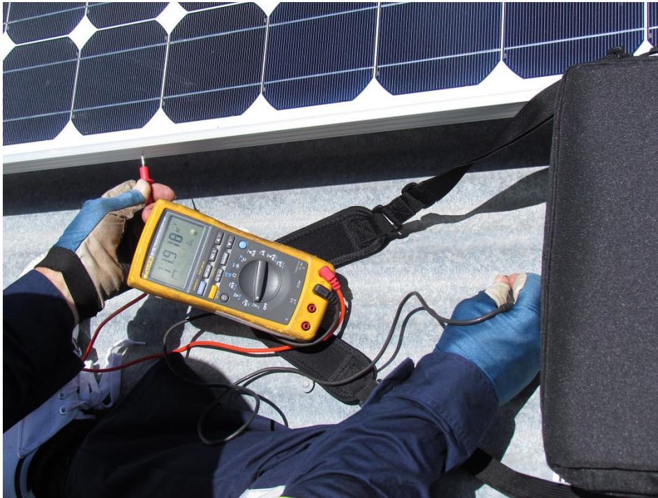
Figure 4: Unearthed PV module frame at potential relative to earth. Although 11.92V is not a hazardous potential, and unlikely to be detected without a Voltmeter, an unearthed PV array can be at a potential different from earth. This particular case was not hazardous when inspected. Under differing conditions and particularly in systems where transformerless PV inverters can cause capacitive leakage currents, missing equipotential bonding of framework and PV array support structures can pose an electrical shock risk.
