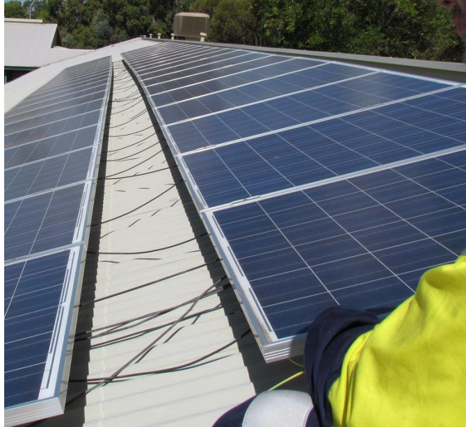
Figure 2: System with inadequate cable protection for PV wiring. This cable protection is needed as heat and especially UV radiation will affect the insulation of the cables. Over the expected lifetime of the PV system (25 years or more), these cables can deteriorate and increase the risk of short-circuits and fire, or will require expensive replacement work, thus affecting the financial return of the system.
