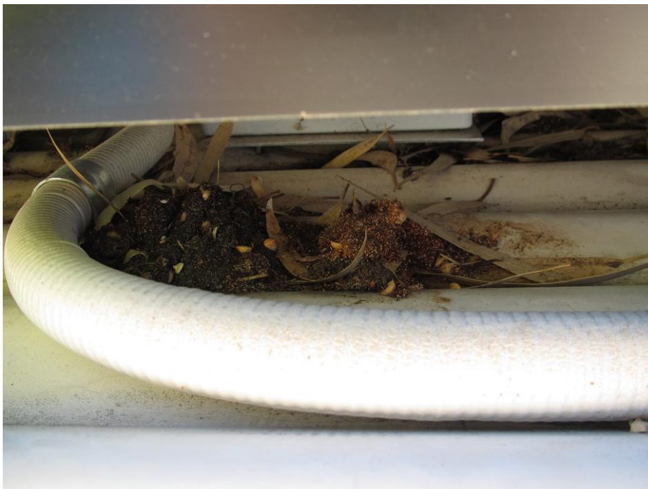
Figure 3: Example of accumulation of leaf litter under PV array panels due to the installation not facilitating self-cleaning. This is of concern because flammable material in close vicinity of a PV array installation presents a fire risk since high resistance faults (caused for example by component failures, bad joints or vermin activity) can lead to arcing.
