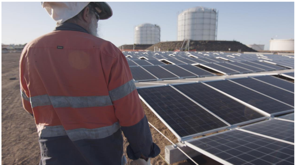
Figure 9. PV is increasingly used for power supply at isolated communities where there can be skills shortages. Novel deployment technologies lower the cost of deployment. Images courtesy of 5B Pty Ltd.
