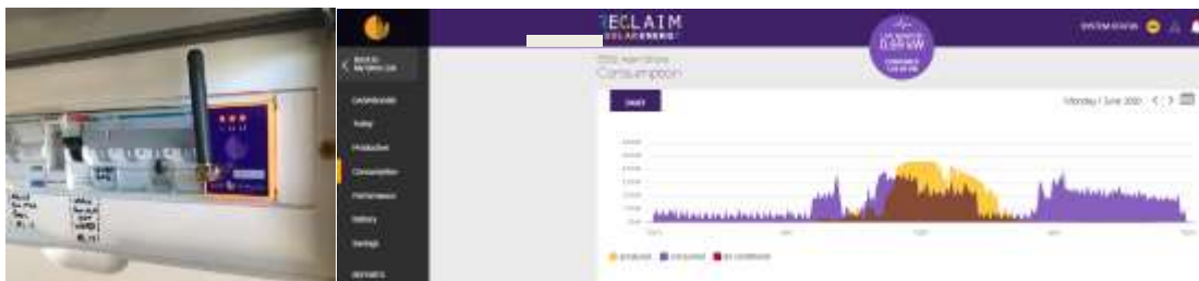
Fig. 2. Solar Analytics installation for a solar PV hot water system: Left, device installation at switchboard and (right) online monitoring platform [5,8]
