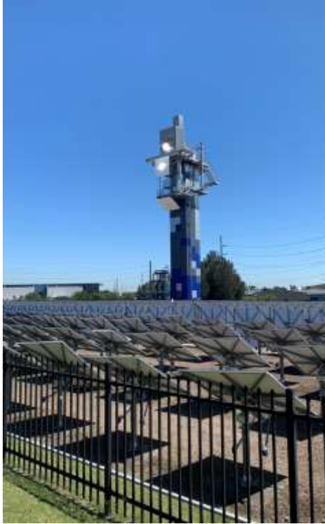
(a) Solar Field 2 with particle receiver system at CSIRO Newcastle
