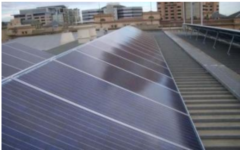
PV modules mounted on a tilted frame on the South Australian Parliament House (Photo: SA Government)
