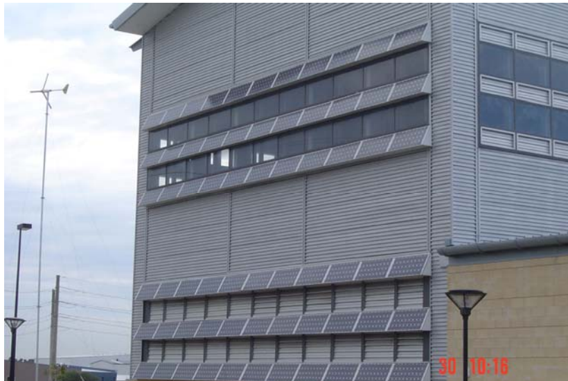
PV Sunshades on the CSIRO Energy Centre, Newcastle (Source: R.Corkish)
